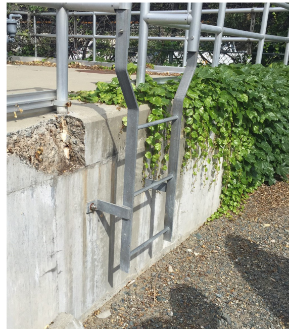
Concrete Repairs are Necessary
