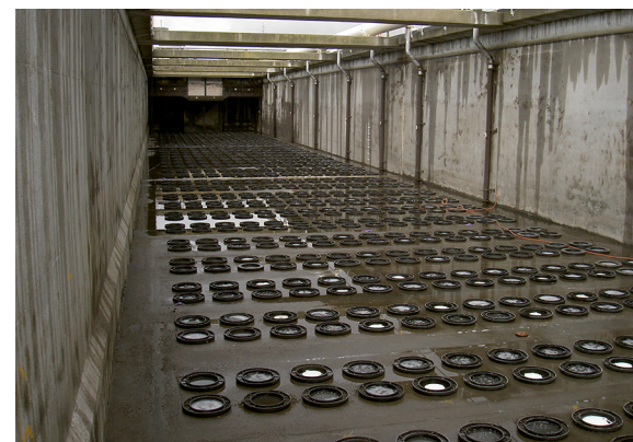
Leaks in Air Piping Need Renovation
