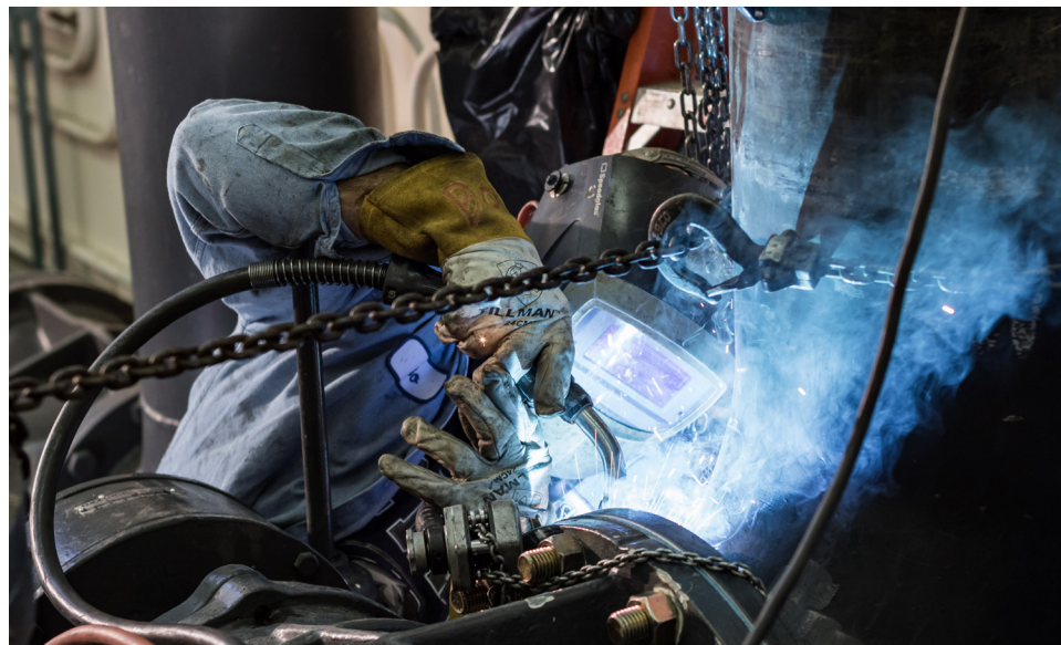
Technician Welding - Ongoing maintenance has helped extend the life of piping and equipment.
