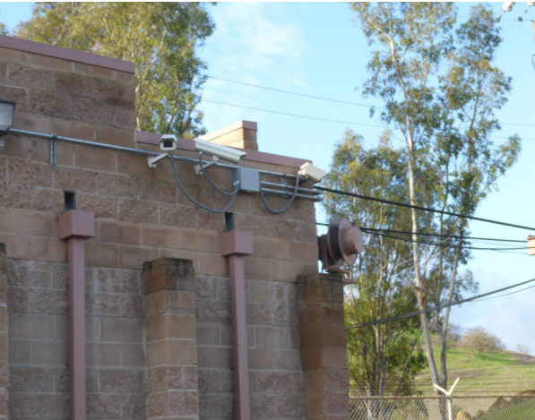
Capital Improvements are Needed for Security
