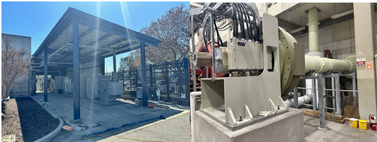
Construction progress for the new electric blowers and transformer facility under the Electric Blower Improvements – District Project No. 100015
