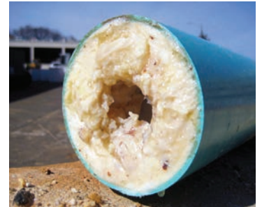
Yep, that's congealed grease clogging a pipe. Gross!
