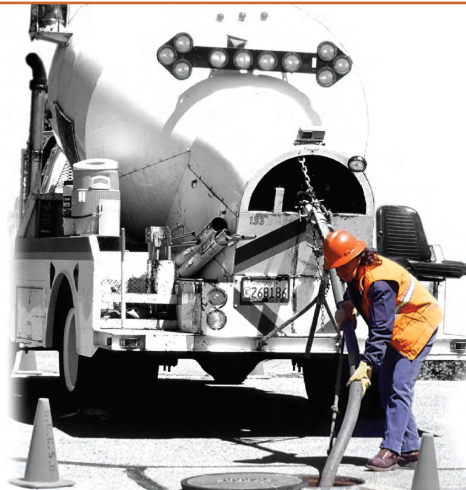
Our crews use specialized technologies, vehicles and equipment to clean sewer pipes every day.
