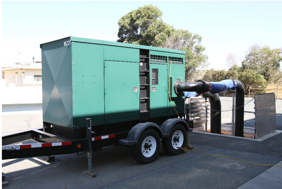
Figure 4.17 Portable Emergency Bypass Pump at Martinez Pumping Station
